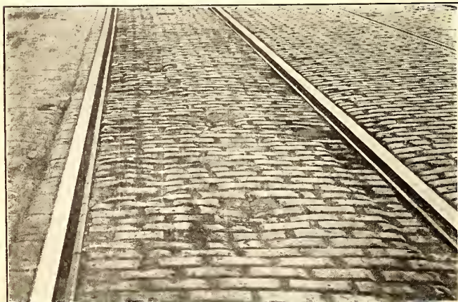
TRACK MAINTENANCE DATA—FIG. 7, SLAG BRICK PAVING SHOWING DAMAGE NOT CAUSED BY RAILWAY
